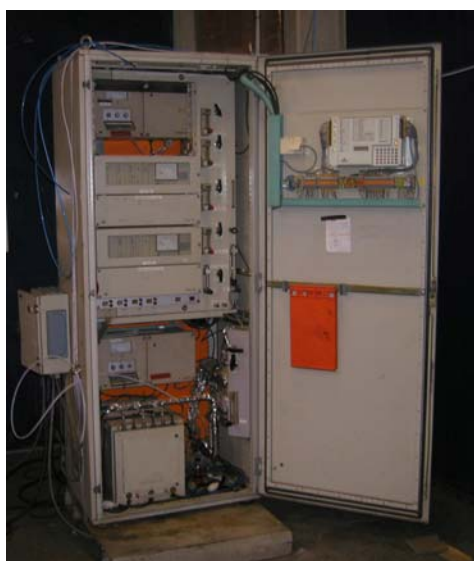
Mobile cabinet with conventional gas analyzers, gas cooler and PLC controlled purge system
